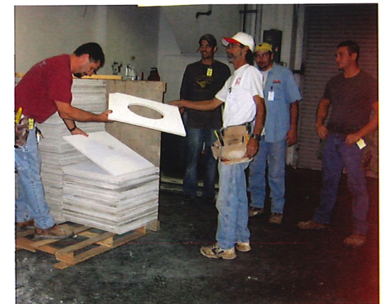
Ken Saunders, Superintendent with Pray Construction and his crew stack ceiling tiles for recycling.
